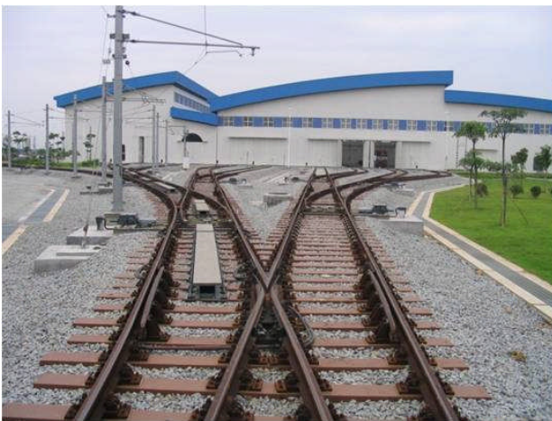
Fig. 11: FFU synthetic wood, switches, at train depot, China
